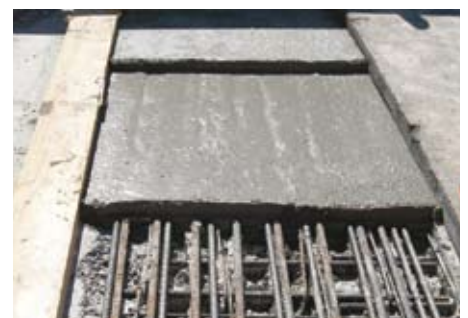
A fine layer of Ductal® is poured, both strengthening and waterproofing the structure
