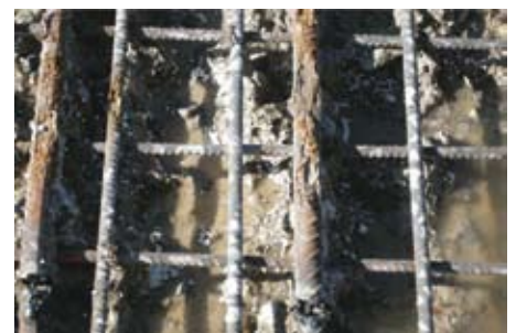
Original state of the corroded reinforcement bars
