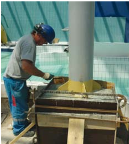
Ductal® is used to renovate the anchor plate of a metal pillar with a badly corroded base
